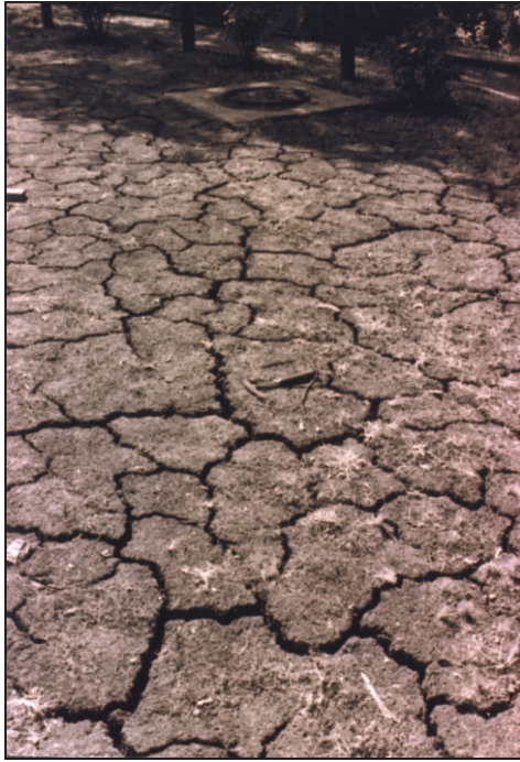
Figure 1: Polygonal pattern of surface cracks in the dry season. These cracks are approximately one inch wide at the top. Note sewer manhole in background.
