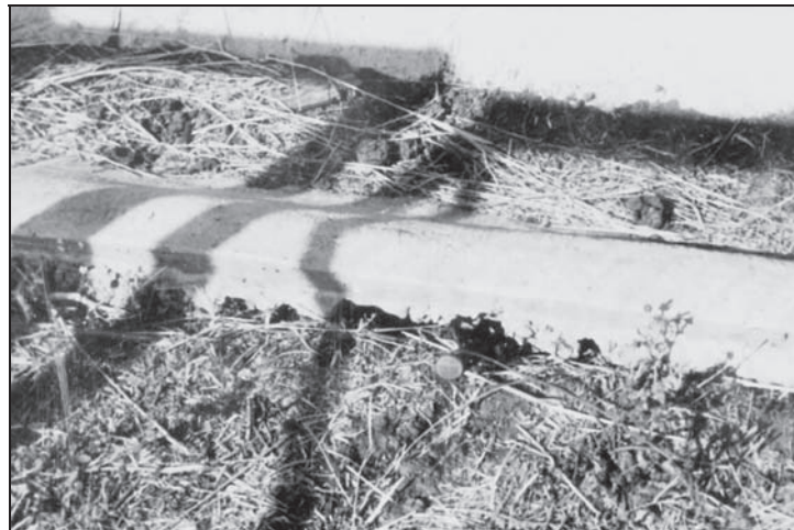
Figure 5: Void created under concrete drainage interceptor ditch by contraction of clay soils.
