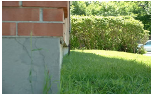
Building damage: note displaced bricks and inward deflection of foundation. U.S. Army Corps of Engineers Photo Click Image to Enlarge
