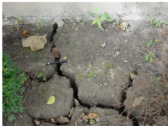
Desiccation cracks in soil caused by drying. U.S. Army Corps of Engineers Photo Click Image to Enlarge
